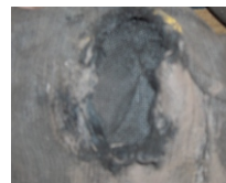
Melted or Charred areas
